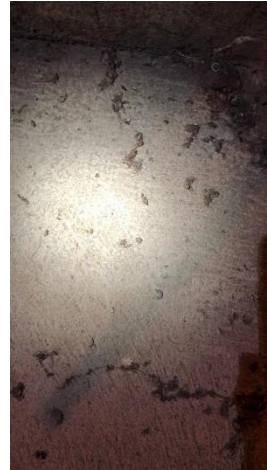
Abb. 3: geringe Kotmenge Pfeiler 1 Ost
